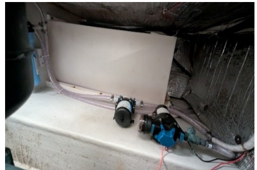
Fresh Water pump and Accumulator tank
