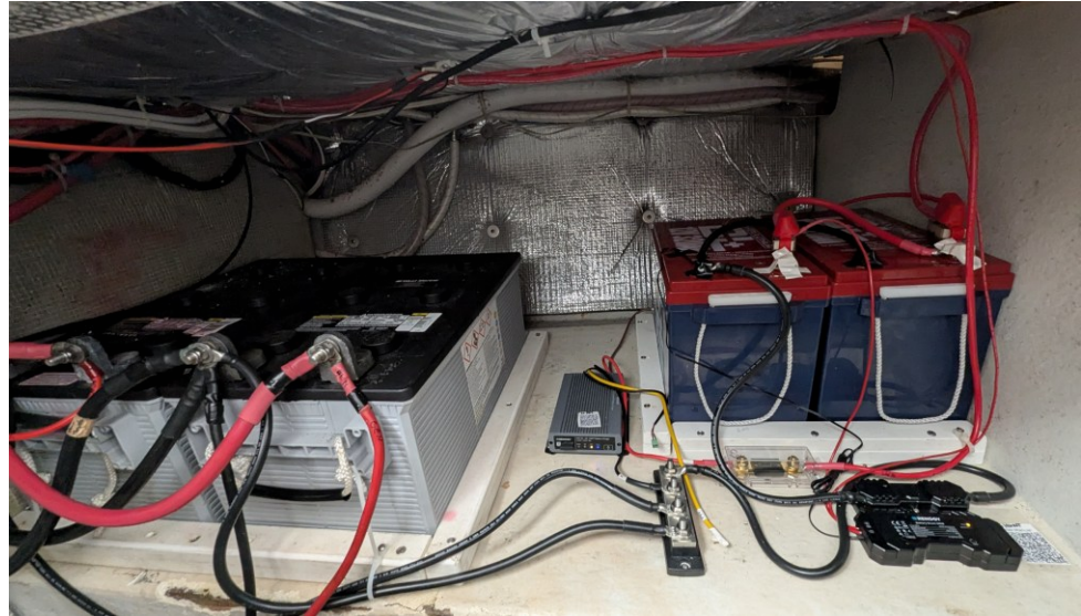
AGM Batteries on the left, LiFeP4 on the right, Note MPPT/DC-DC charger between the batteries and the DC Shunt in the Lower Right
