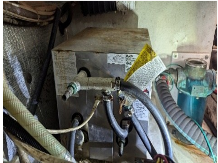
Note, the hot water outlet is not connected to anything.
