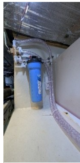
Water Filter, Note By-Pass in the upper left
